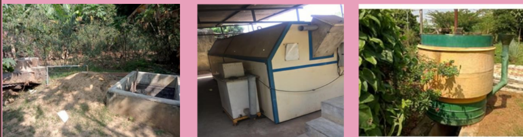
Bio compost & bio gas unit
