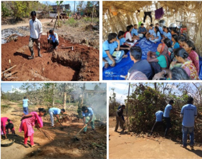
Restoration of water and sanitation post Cyclone Titli in 5 villages of Gajapati, Odisha Post Titli Cyclone
