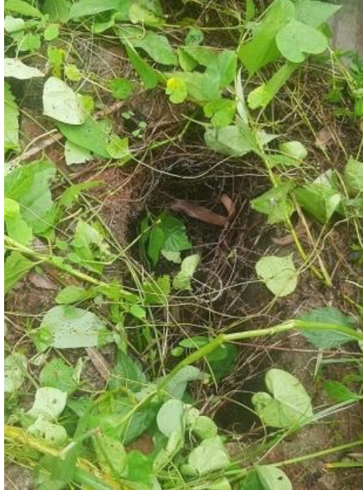
(Transformer Earthing Point)
