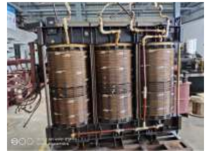
Inside View of Power Transformers
