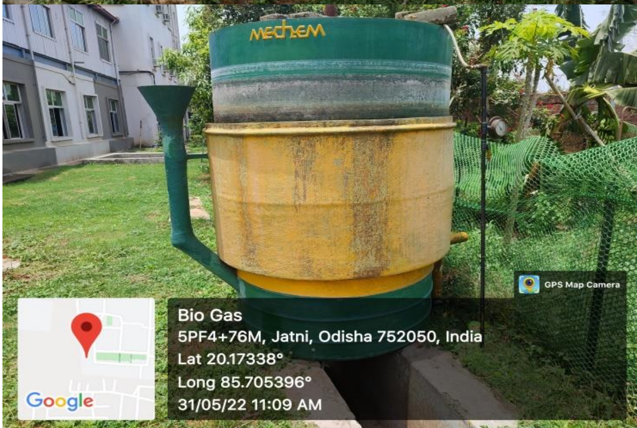
Fig. Biogas Plant
