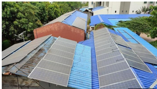
Solar Microgrid Centurion Market Complex
