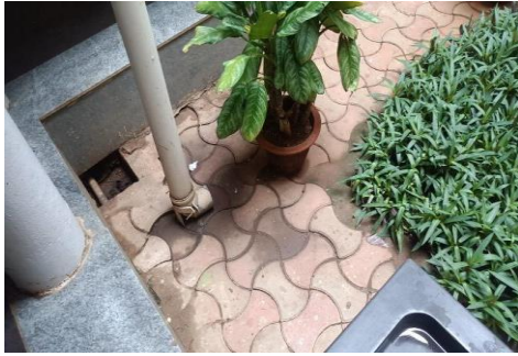
Rain Water Harvesting Point-01
