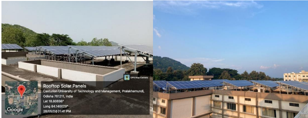
Solar panels fixed in the Top of the Building
