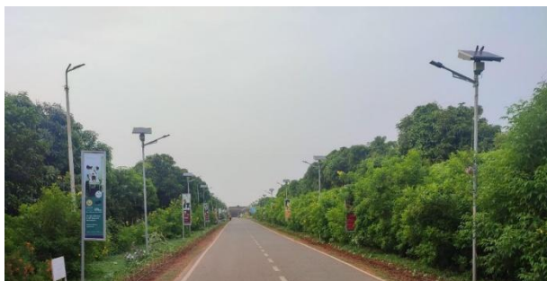
Solar Street Lights Installed inside the Campus
