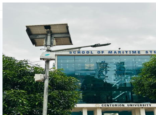
Aurasure system installed inside the Campus
