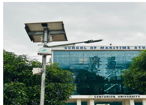
Solar operated Controller
