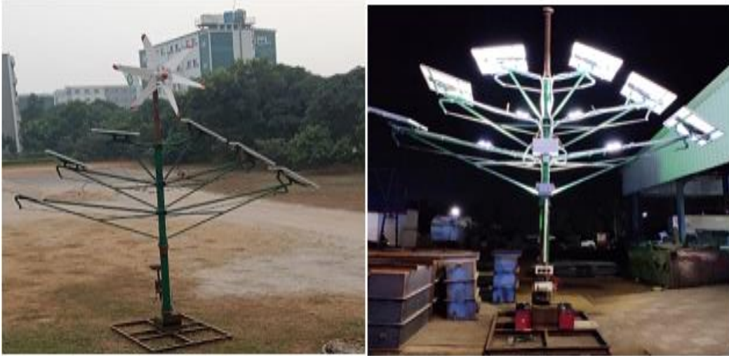
Fig.101 Solar Lighting at University
