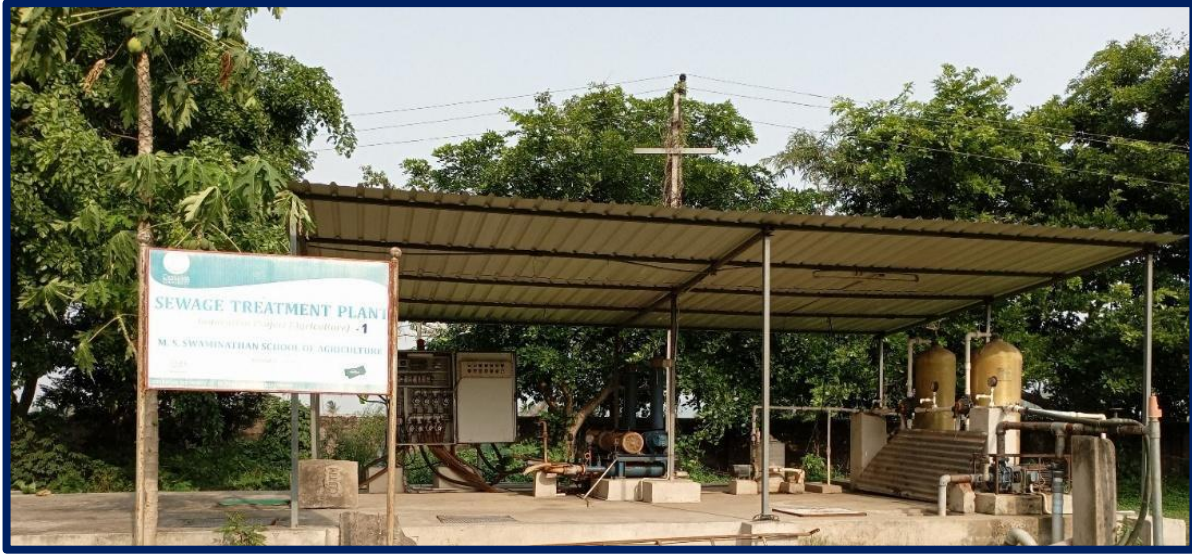
Fig. 29 Sewage Treatment Plant
